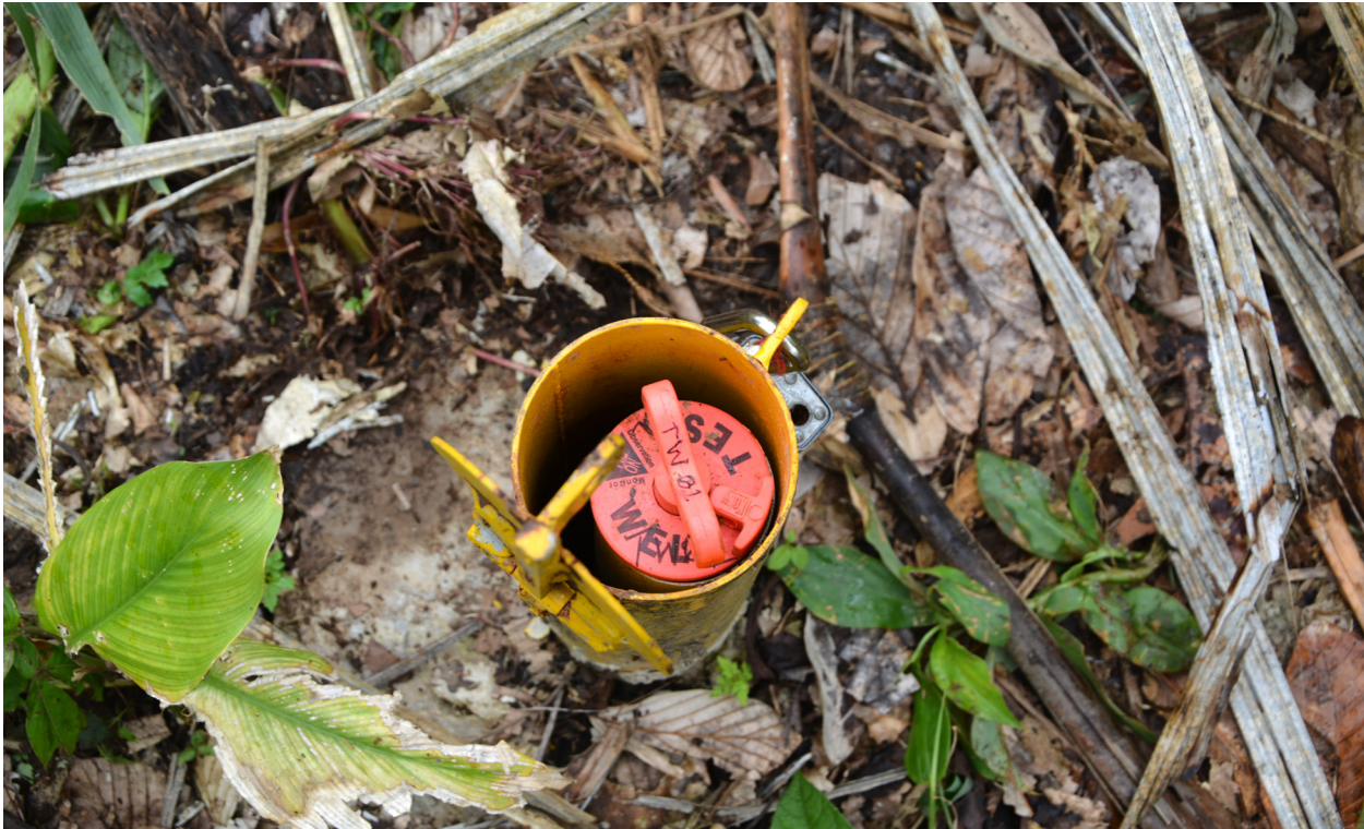
Aguarico 6, June 2015, catchpit and water monitoring well, used to measure the contamination of underground waters and soil.
